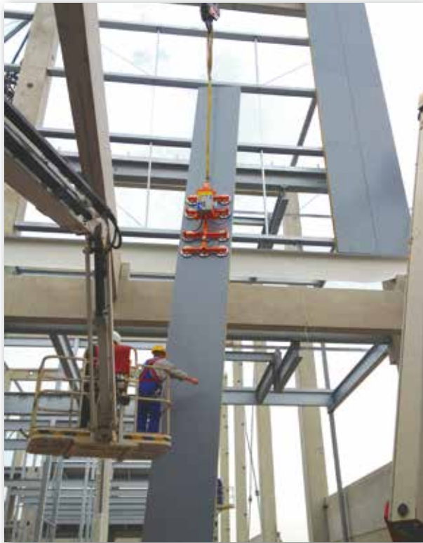
Vacuum based installation of 12 m long wall panels with the OKTOPUS® PANEL-Jack KS-B
