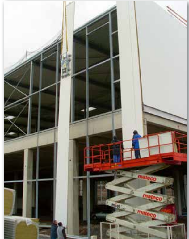
The photo shows the installation of 17 m long elements with the OKTOPUS® PANEL-Jack KT-B .
